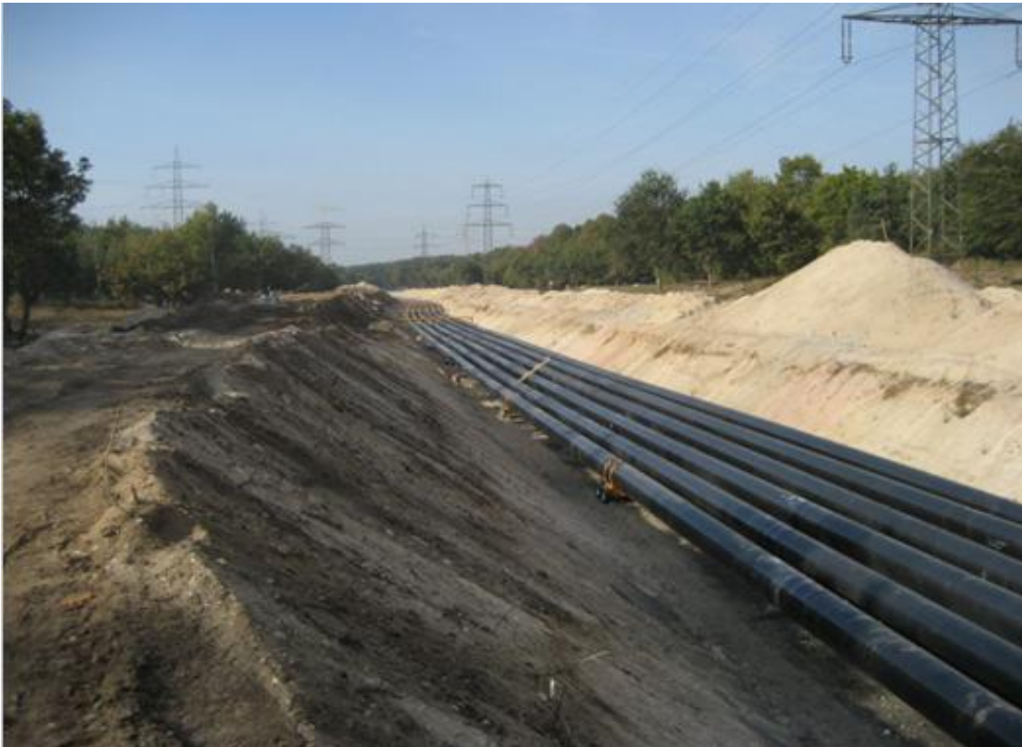
Figure 9: Example of direct buried gas insulated line prior to backfilling – Frankfurt Airport
