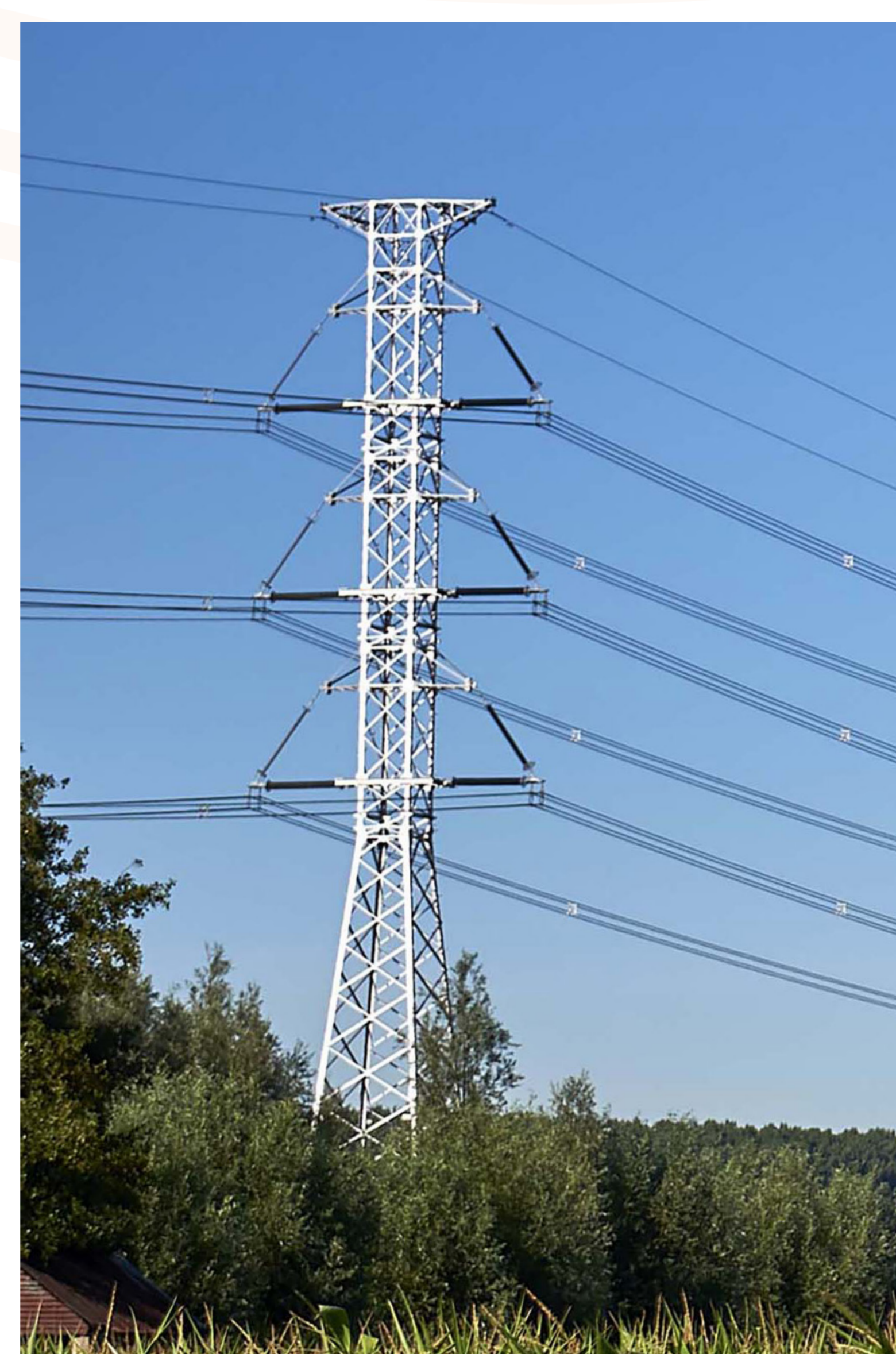
'Compacte' mast 380kV
